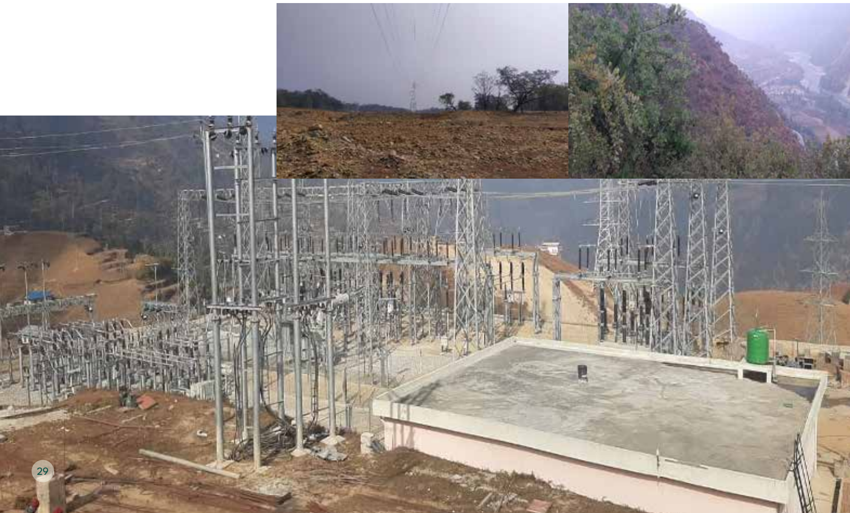
Sunkoshi River Crossing by proposed CP-1 TL Route Alignment ↘ 132kV Transmission Line Crossing Near Lamahi Substation ↙ Tingla Hub Substation ↘
